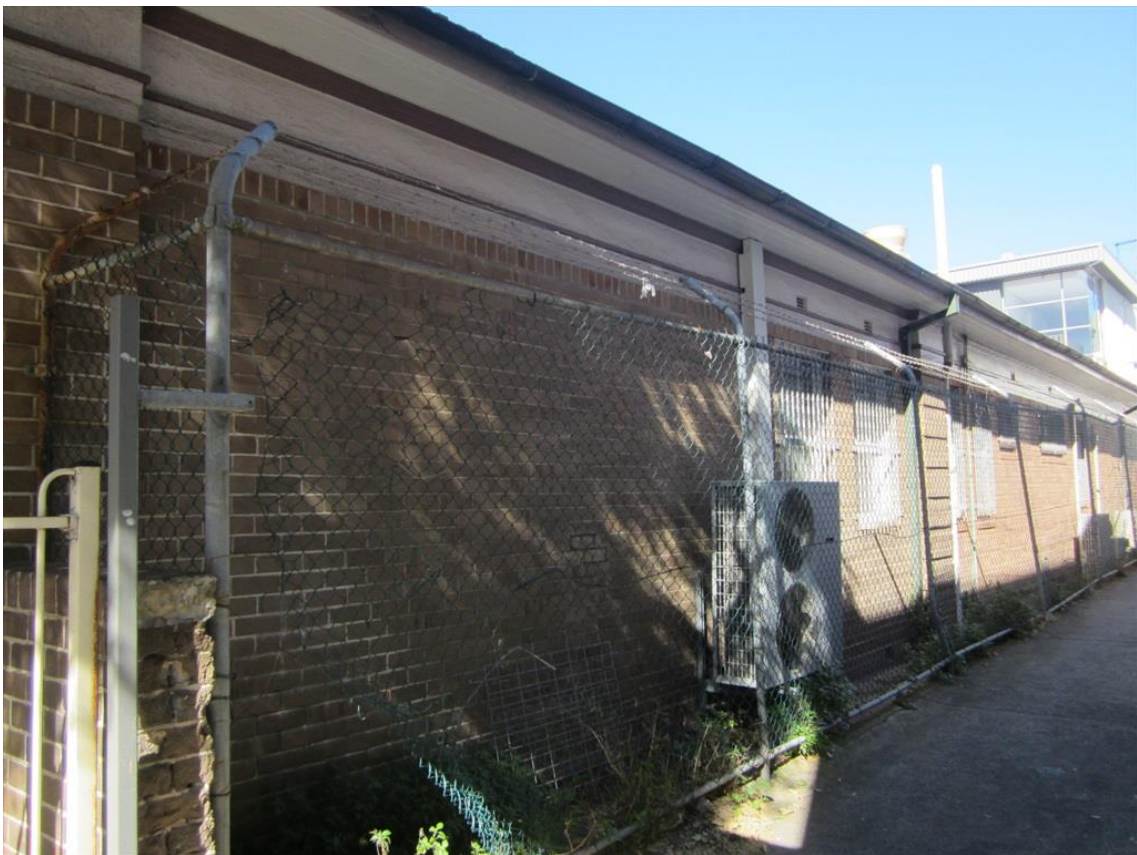
Figure 40 View along the west façade; the rusticated pier indicates the extent of the c. 1934 addition
