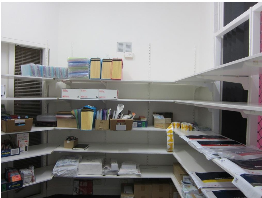
Figure 45 Interior of the north-east porch, now store; the entry is infilled (right of image), the entry to the phone booth is infilled (centre) and later door opening to the retail space (at left)
